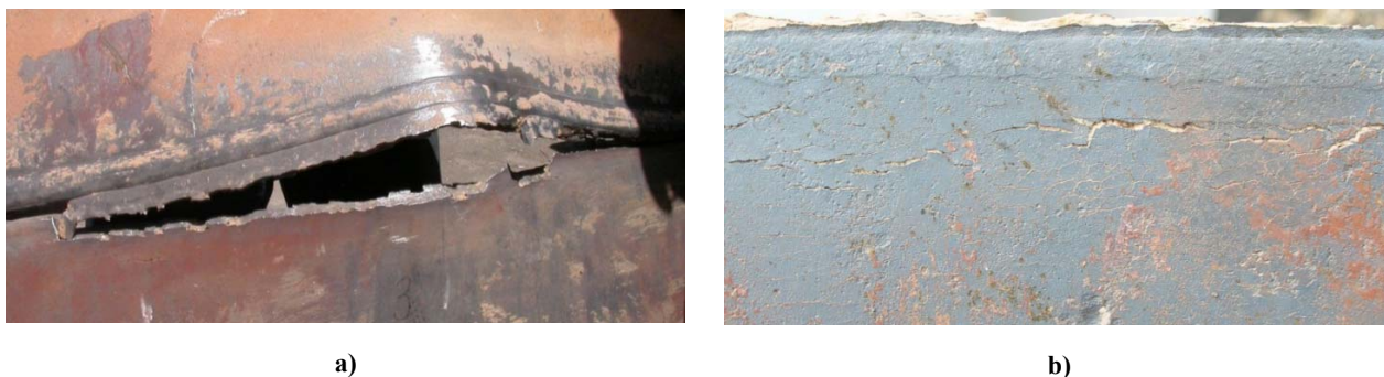
Fig. 4. Destroyed pipe with crack (a) and net stress-corrosion cracking (b) along the factory weld seam
