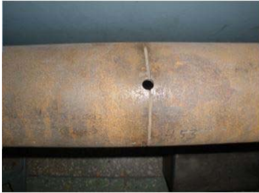
Fig. 2 Sample pipe, defect II: notch with a hole
