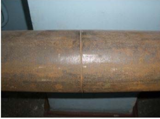
Fig. 1 Sample pipe, defect I: notch
