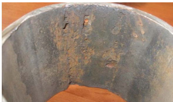
Fig. 2. Internal corrosion damages fragment pipeline pipes category X60
